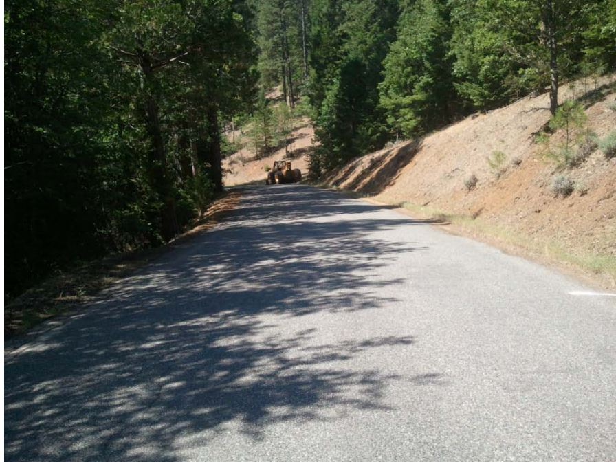
Figure A-13 Section 3, Location 8. Road width is 20 feet, with east and west shoulder widths of 2 feet. Grade is 1.7%.
