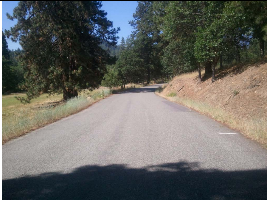
Figure A-10 Section 3, Location 4. Road width is 23 feet, with east and west shoulder widths of 0 and 3 feet, respectively. Grade is 0.6%.
