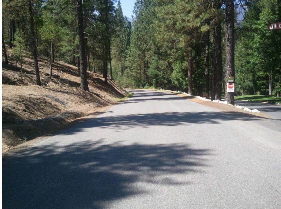
Figure A-19 Section 6, Location 0. Road width is 19 feet, with east and west shoulder widths of 2 feet and 1 foot, respectively. Grade is 4.5%.
