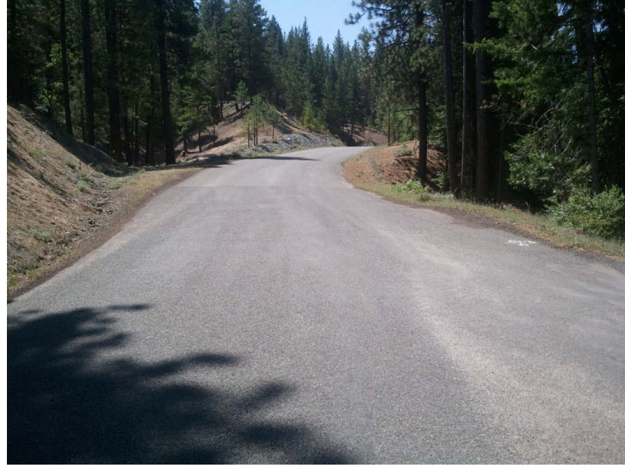
Figure A-21 End Section at intersection of French Creek Road and Homestead Lane. Road width is 22 feet, with east and west shoulder widths of less than 1 foot and 2 feet, respectively. Grade is 7.6%.
